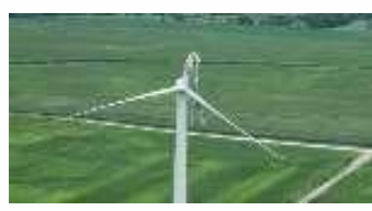
Wind Blade Damage by Fierce Storm
