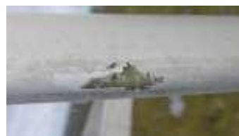
Topcoat due to Air Trapped in the Manufacturing Process
