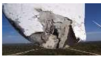
Blade Tip Damaged by Lightning Strike
